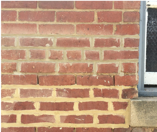
New mortar does not match the historic mortar in color or tooling.
