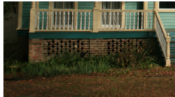
Recessed pierced brick lattice retains the visual qualities of the brick pier foundation.
