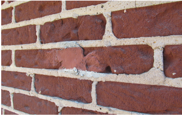
Sandblasting can irreversibly damage masonry.
