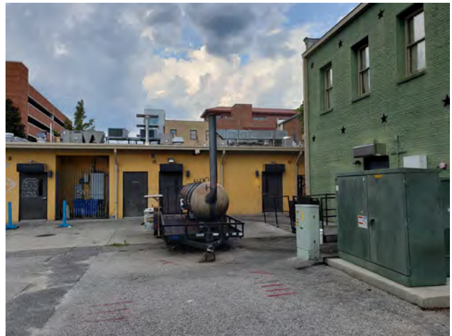
Above: Rear Elevation of 30 N Main Street as viewed from the south.
